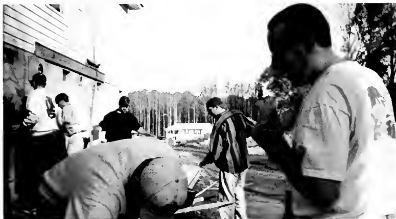
Hard At Work ... Carl Osberg said, "My brothers and I enjoy participating in Habitat for Humanity. I feel good after being able to help build a house for those in need."
